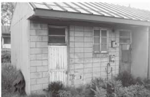
▶老朽化が進む町営住宅
